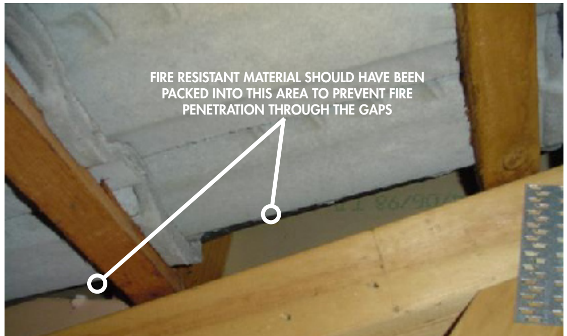
An example of a fire separating wall inadequately finished around roof battens to the underside of concrete roof tiles.
